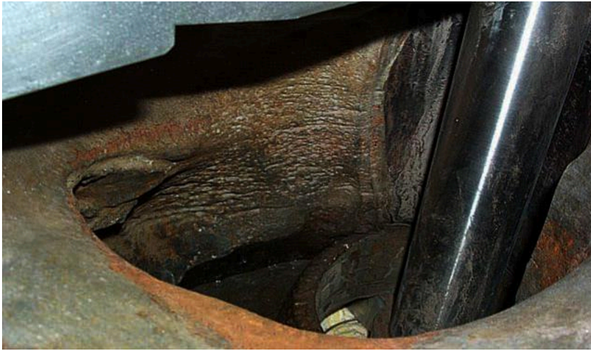
Example of corrosion by "electron stripping" in Cleveland nuclear plant.
