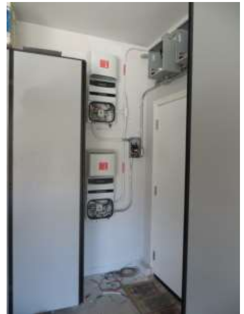
Figure 7 Inverter Sub-panel and DNA Filters
